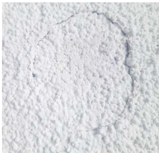
Fig. 3. Coating damage after hard body impact
