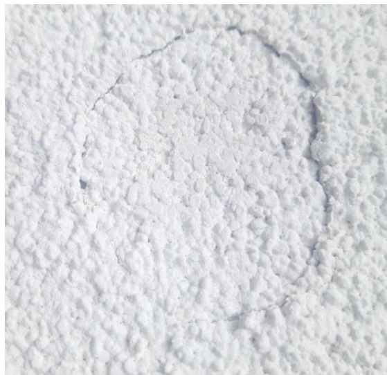
Photo 1. Coating damage after hard body impact
